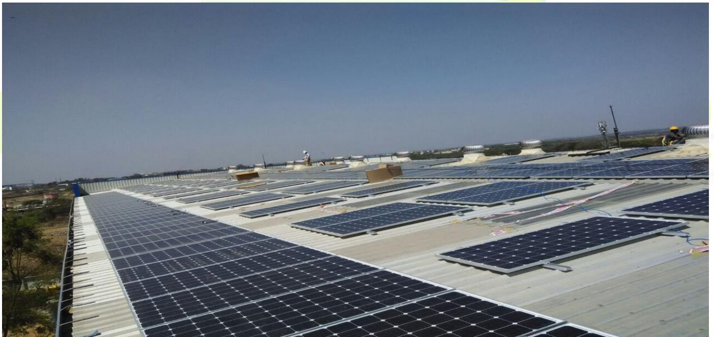
160 Kw @ BHEL, Secunderabad, Telangana
